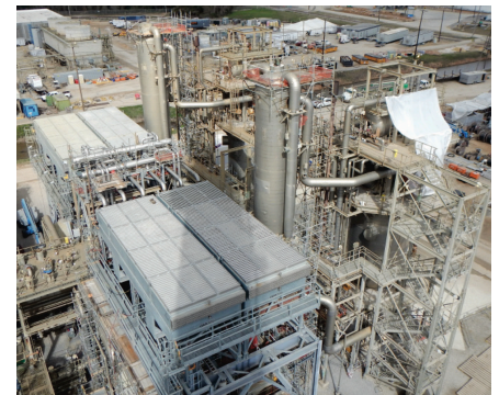
Modern view of the Beaumont methanol plant (now owned by OCI)
